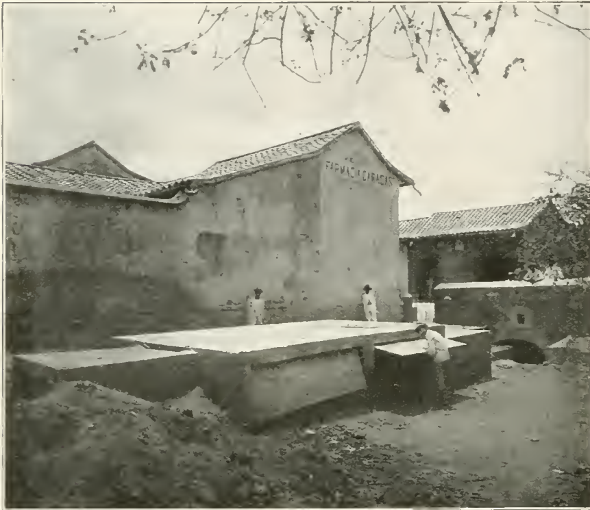
Discharge gates for flood water peak loads. Where rain falls at times at the rate of three inches per hour, the overflow discharge is very rapid.
